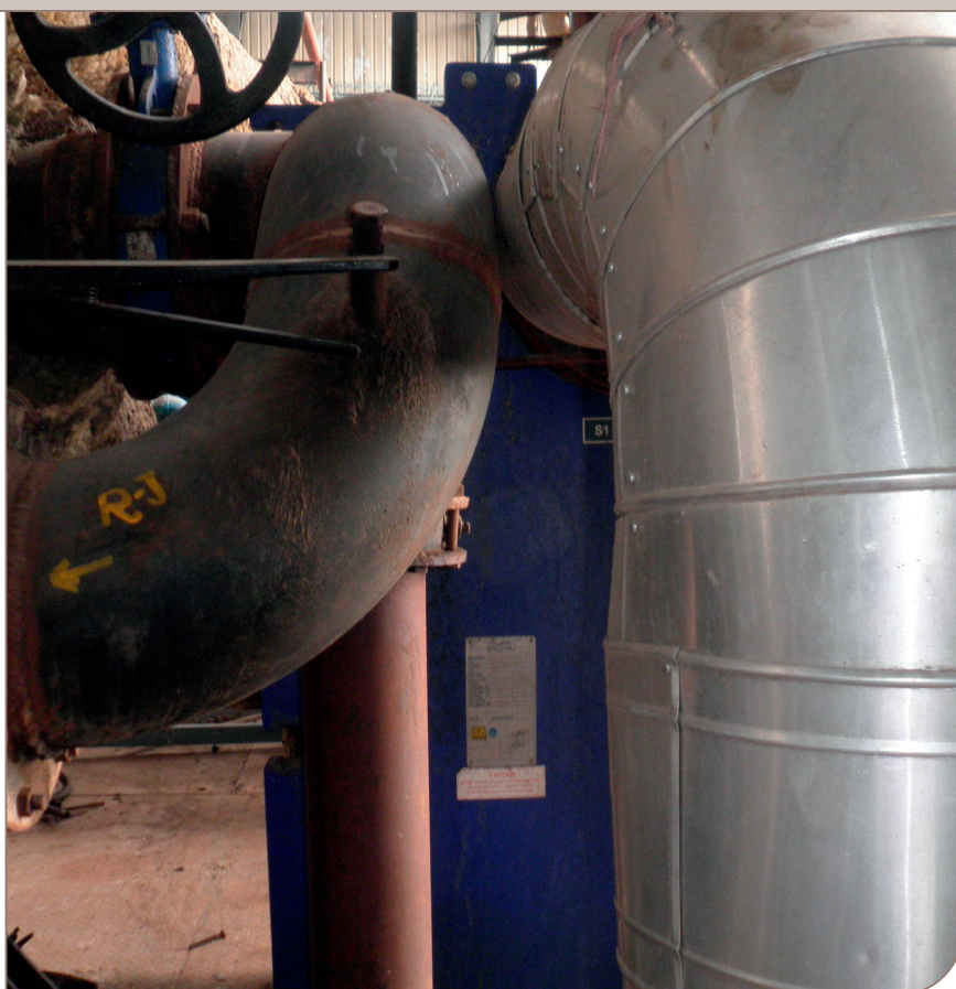
One of four Alfa Laval WideGap PHEs installed at Shri SaiKrupa for heating raw sugar juice.
